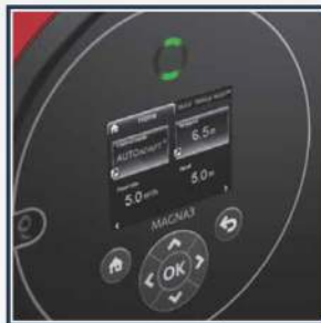
Data FLOW Meter (MAGNA3 Grundfos water pump) (installed on output pipe)
